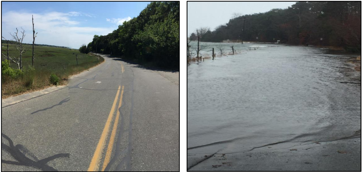
Figure 2. Calm and flood conditions along Samoset Road. Frequently inundated sections of roadway are at imminent risk of failure.
