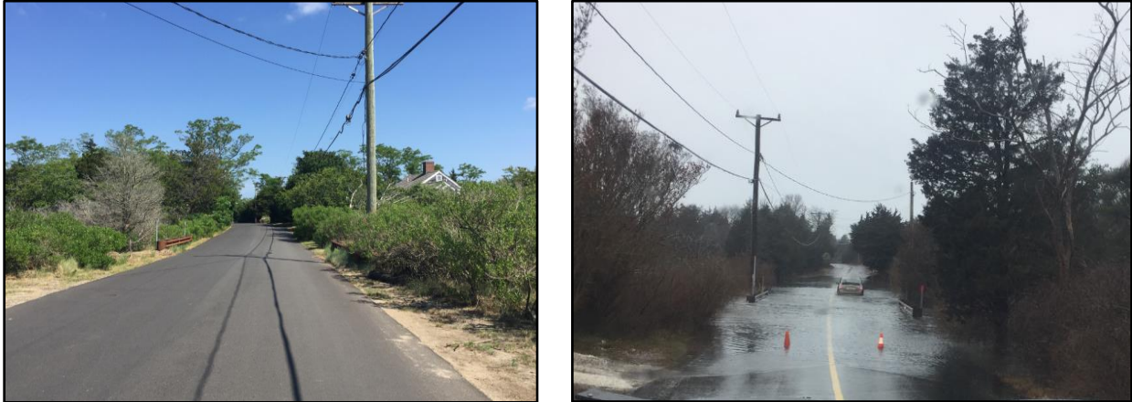
Figure 4. Calm and flood conditions along Dyer Prince Road. Roadway particularly vulnerable to flooding adjacent two existing culverts.
